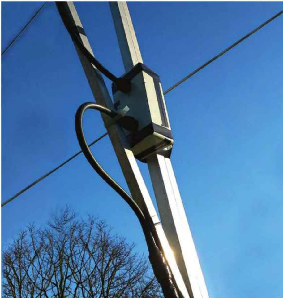
PHOTO 2: Prototype preamplifier weatherproofed and mounted on the Yagi itself.
